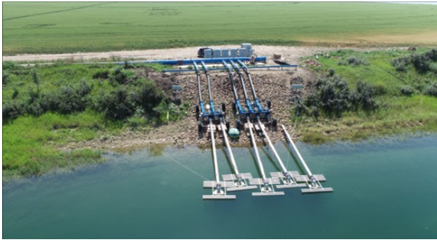
Figure 1 – Seasonal Irrigation Pump Station Mounted on Wheeled Carts within Lake Diefenbaker bed, bank and boundary.
